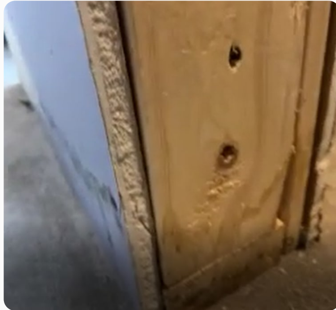
Discoloration was noted on the drywall where the water level was present during the flood
