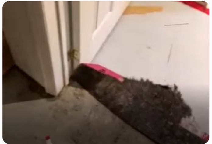
Problematic area under the floor. Possible trapped moisture.
