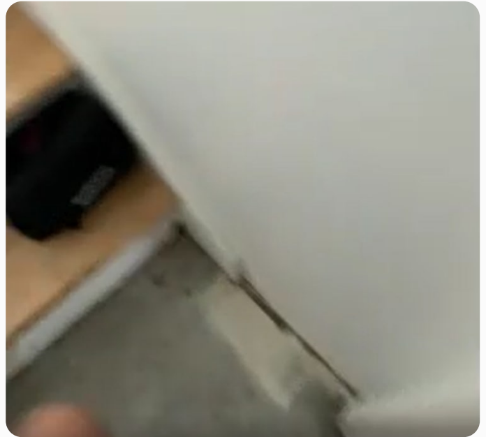
Discoloration and water damage were observed on and by the stairs
