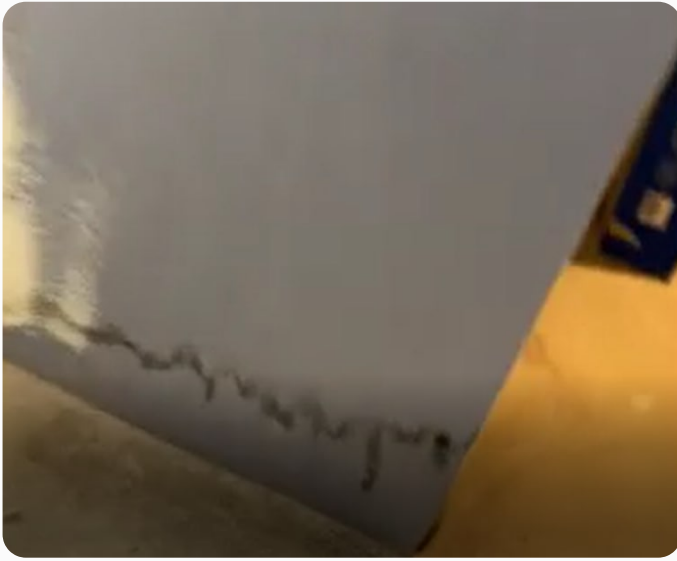
Water damage was noted on the wall
