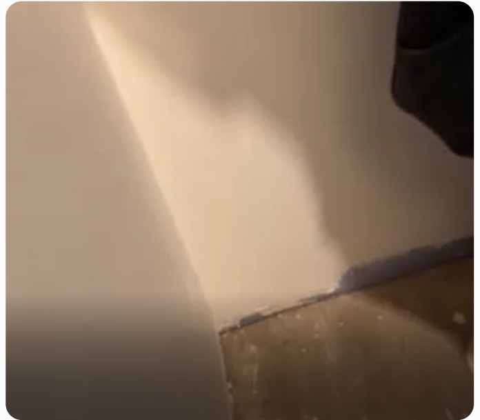
Discoloration was observed in the corners
