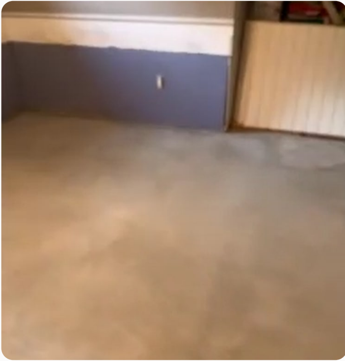
Sump pump is located in the corner
