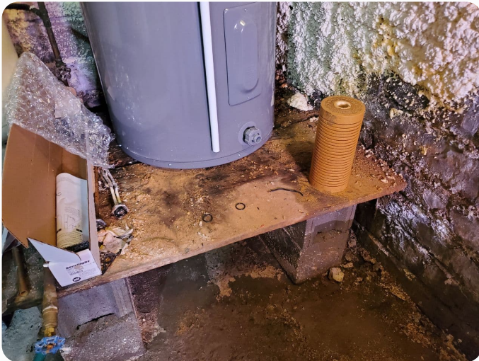
Visible discoloration noted along the wood material
