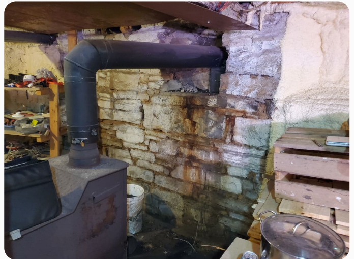
Visible mold growth observed on the foundation walls
