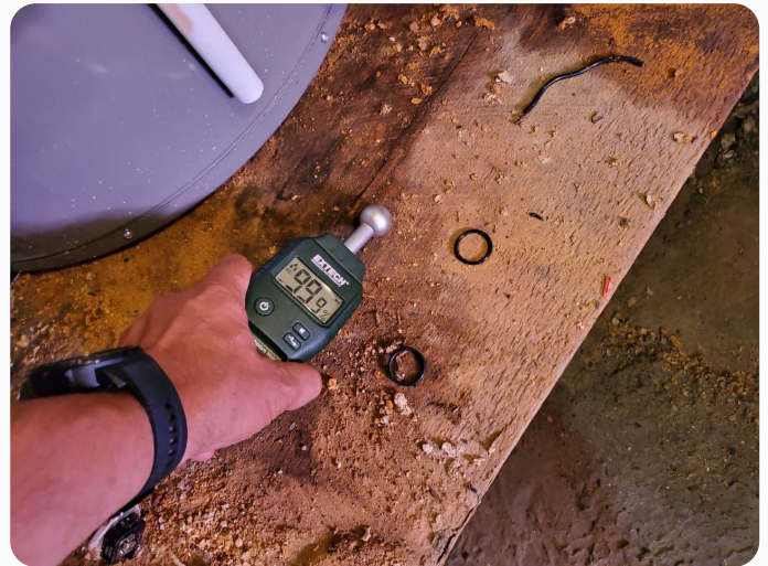
Wooden components affected by moisture around the water tank
