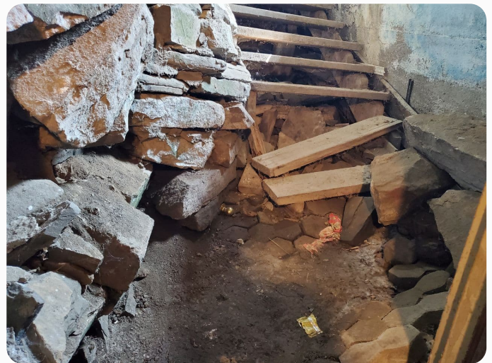
Compromise to the stairs noted; entrance to the basement area
