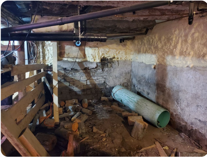
Accumulation of firewood & debris noted throughout the basement area; visible mold noted on the walls
