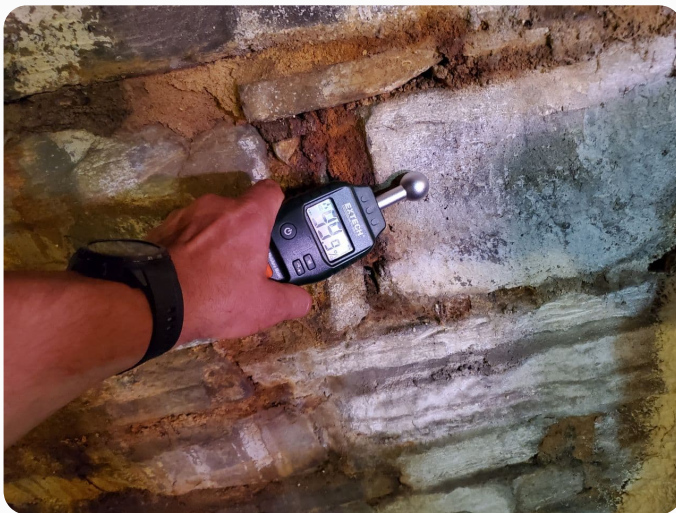
Active moisture content detected along the foundation walls in the Basement Area
