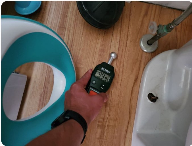
Active moisture detected around the toilet; main level
