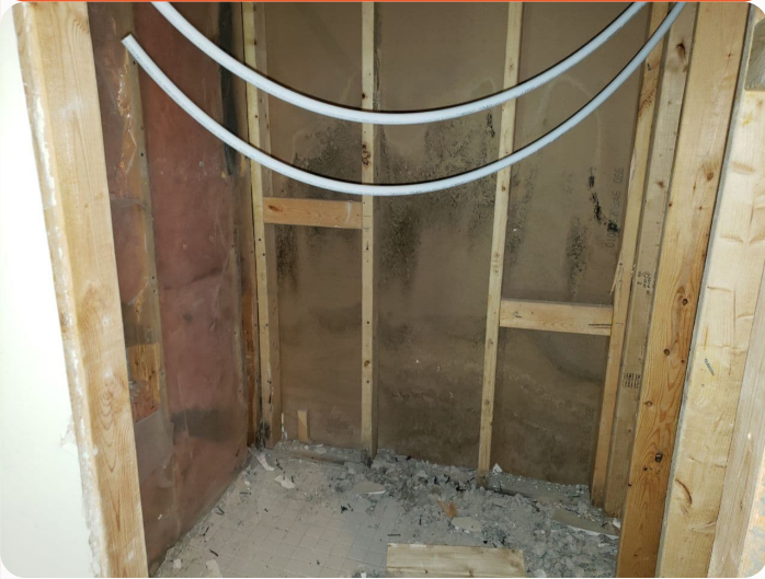
Post-Remediation Verification: August 19, 2022;; Visual mold observed on the wall behind removed shower
