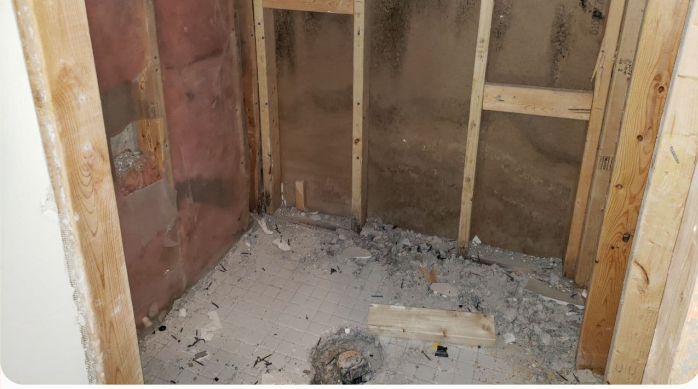
Post-Remediation Verification: August 19, 2022; Shower area found to be in the renovation process at the time of the assessment
